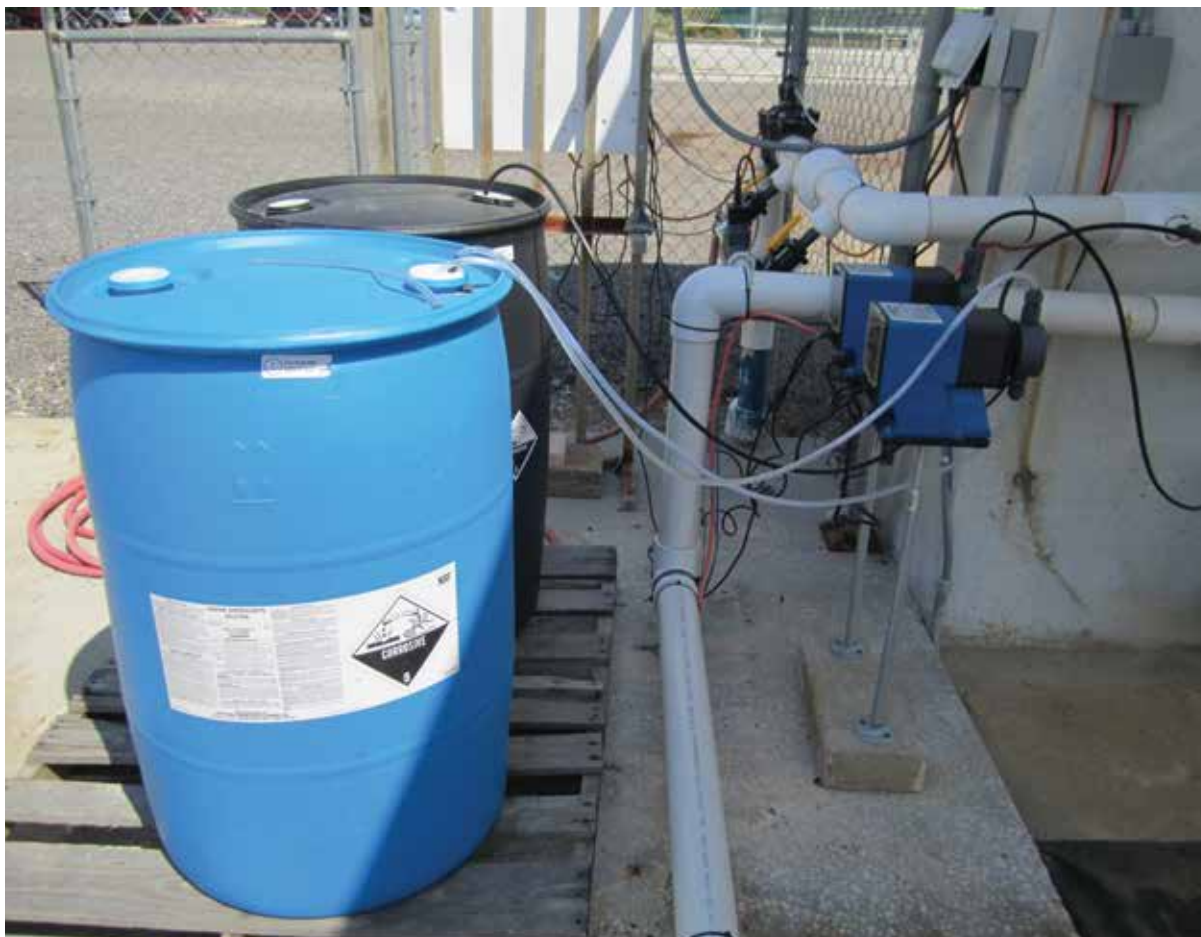
Figure 2a. Liquid sodium hypochlorite.
